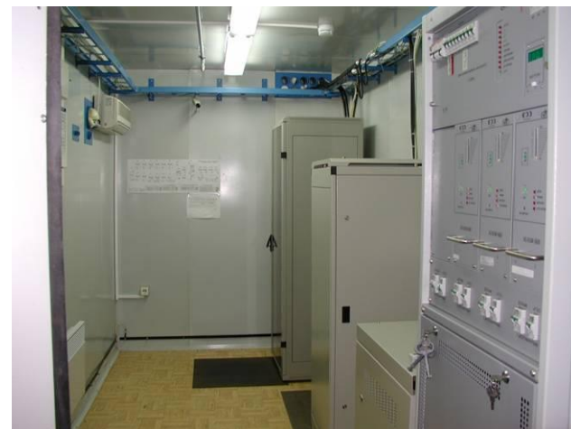
Yaroslav Control Room Center
